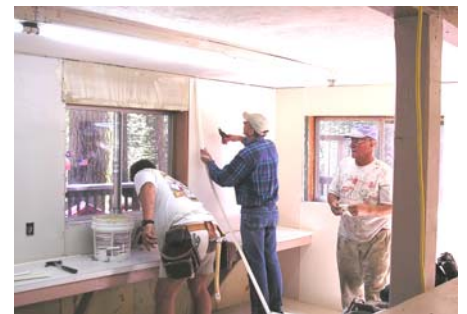
Jeff Koester, Frank Jackson and Bob Paden installing fiberglass reinforced plastic panels
